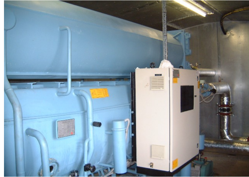
Above – Absorption Cooler Left – Gas fired CHP Engine
