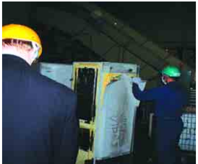
Exhibit D.30 Manual removal of aluminium heat shield from back of fridge/freezer at Green Cycle plant
