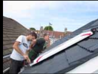
Solar water panels (grant assisted)
