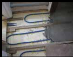
Under floor heating
