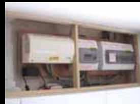
V phase unit and Ultra Eco Units
