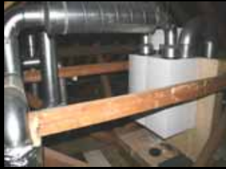
Heat recovery system
